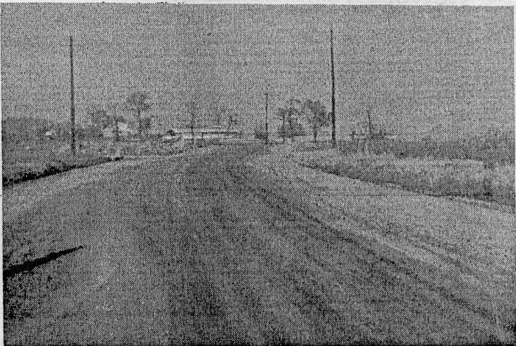
THIS SHOWS the start of grading on Monroe Manor Road looking north from the vicinity of Lot H-27. The low roof on the right is the boathouse.
